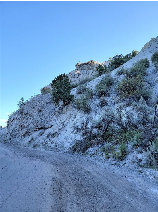
Photo 5. Steep slope with weakly cemented surficial soils
